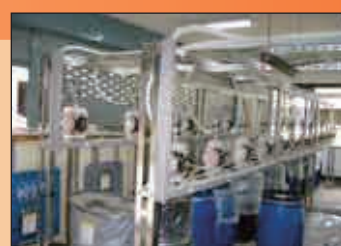
Pump Feed Chemical
